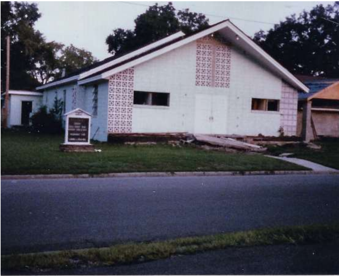
July 1986 – A last look at the old building as it was torn down July 26, 1986.
